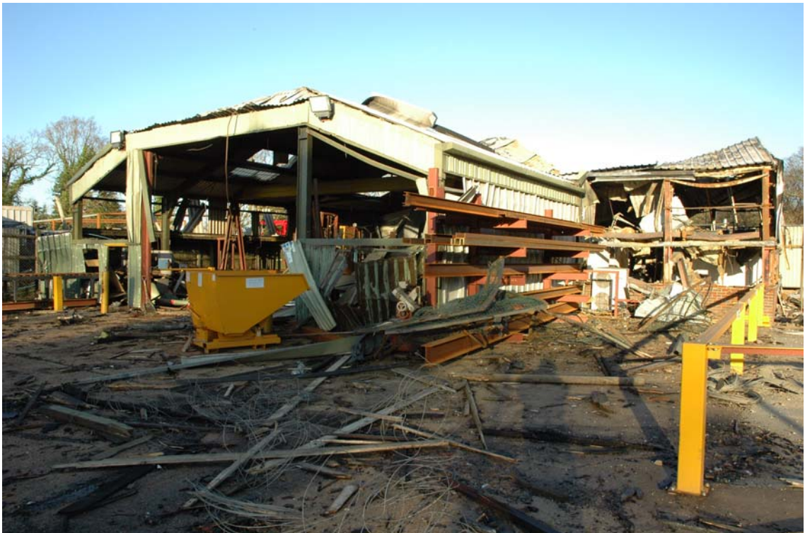
Damage on site to Builders Beams 1 building
