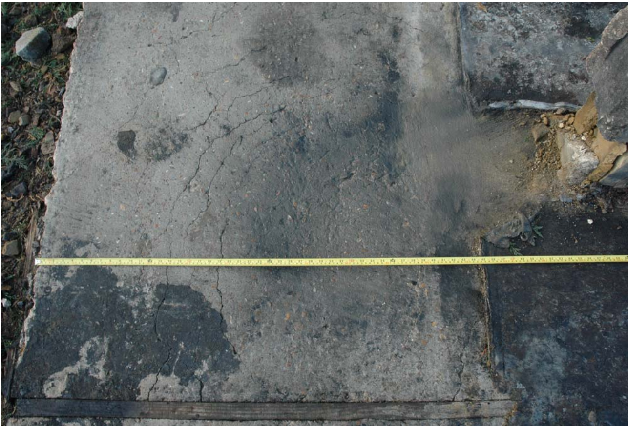
Image showing depression and cracking in concrete walkway.
