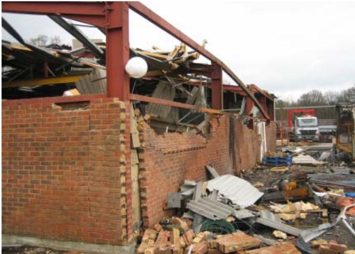
Damage on site to Builders Beams 2 building
